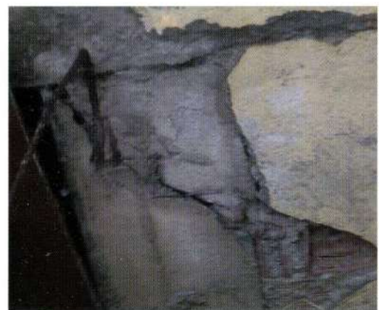
Figure 2: (a) Apparent oblique cracks in the windows "of the market city building", Colonel Amirouche Street of the Ain el Hammam (b) Networking cracks of a house.
